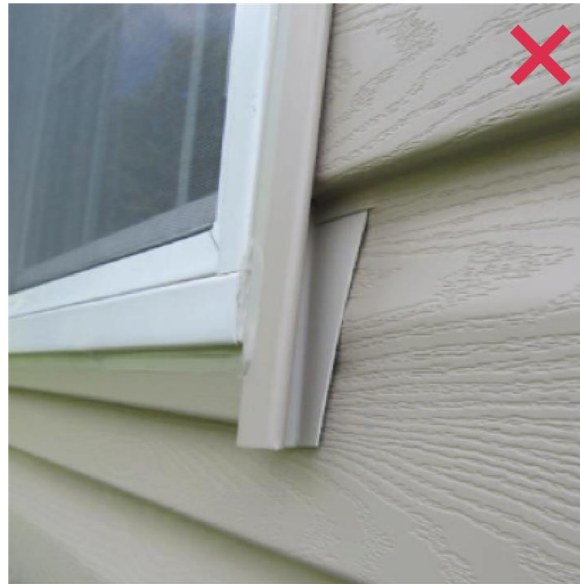
Figure 6: J-channel siding trim at the edge of an off-shelf clapboard cladding system prohibited. Proper trim required.
