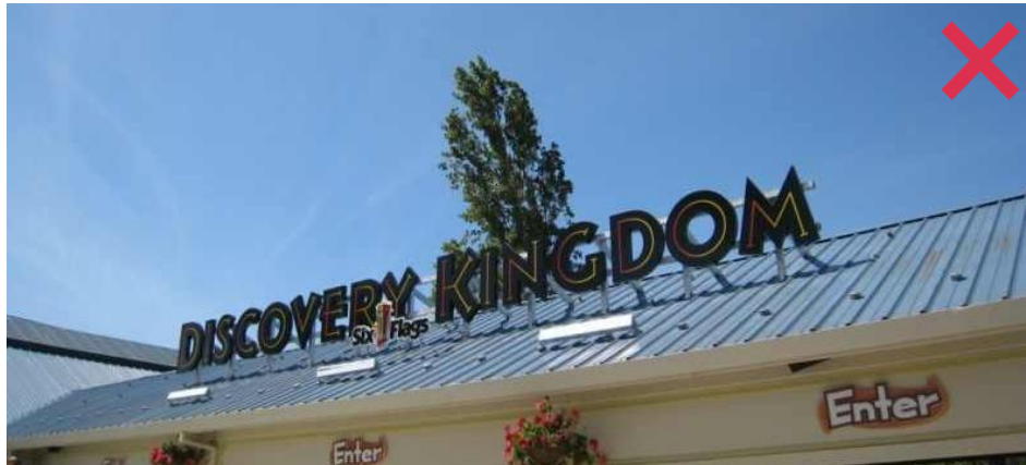
Figure 37: Example of wall sign that is inappropriately mounted on a track and not recommended.
